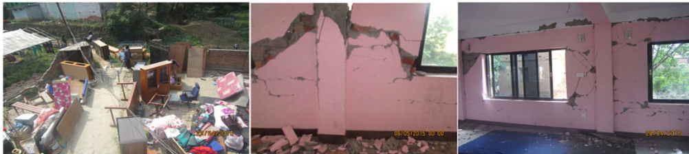
New Life Missionary Training Center Building 's situation after the Earthquake
